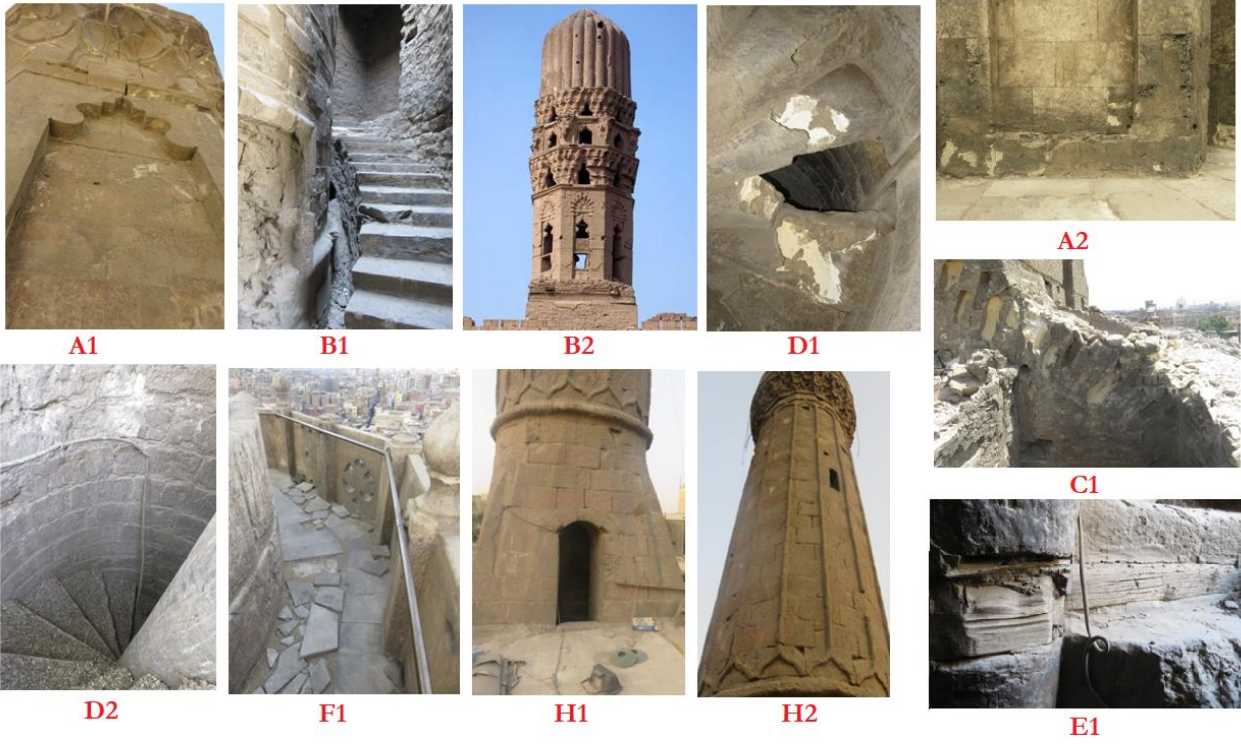
Figure 7. Different levels of present deterioration of minarets' parts
